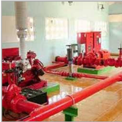
Fire Hydrant System
