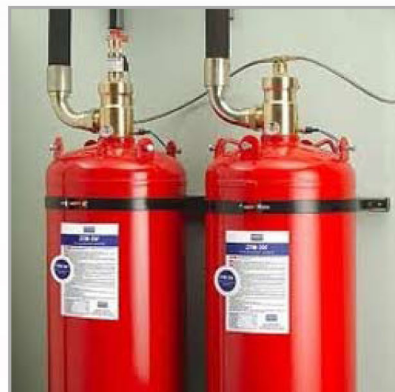
Gas Suppression System
